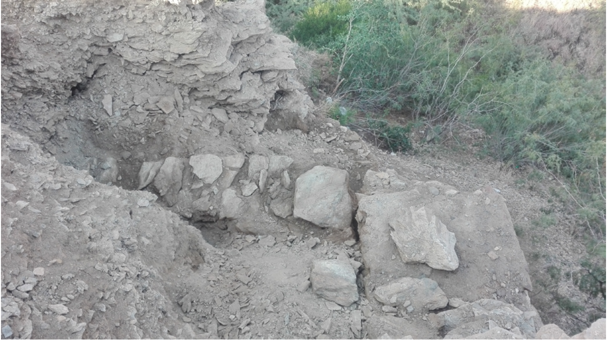
Figure 10. Rubble masonry wall at the north-western corner of Block B1. Due to the threat of potential collapse of the entire retaining wall on the north and west of the corner, it was not possible to go deep to expose clearly the whole wall for proper photography. (Photo: author.)
